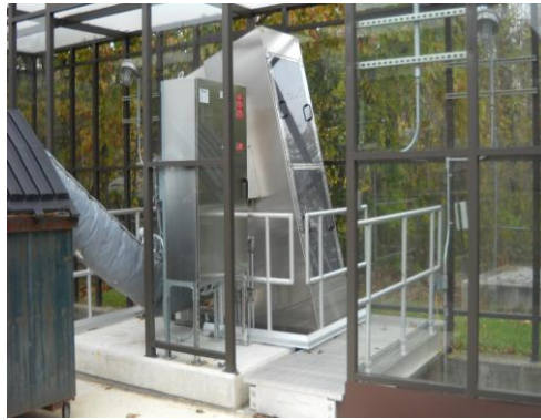
Raw Sewage Screen
