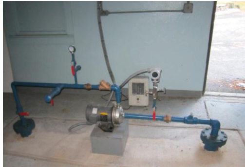
Well No. 2 Modified Pump Arrangement
