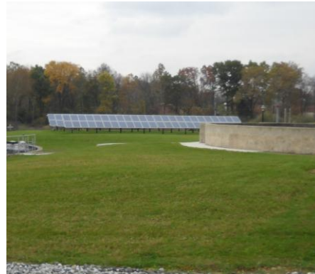
Solar Panels at WPCP Site
