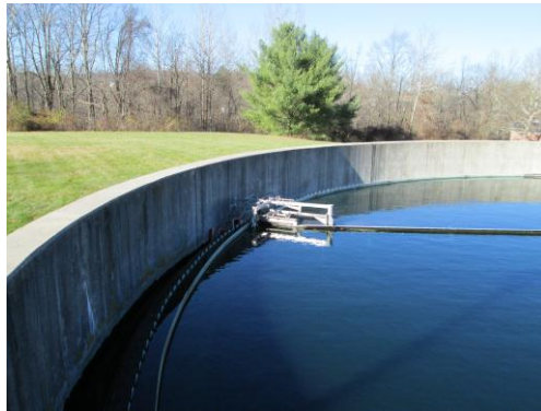
Final Clarifier – Weir Brush System
