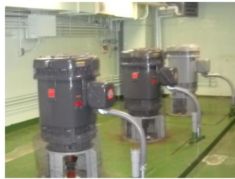
Raw Sewage Pump Motors
