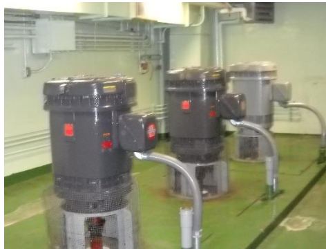
Raw Sewage Pump Motors
