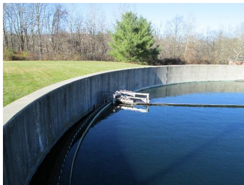
Final Clarifier – Weir Brush System
