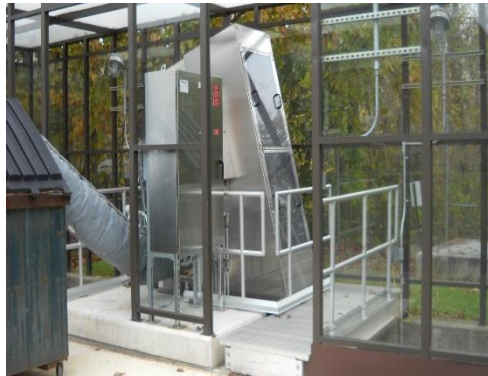
Raw Sewage Screen
