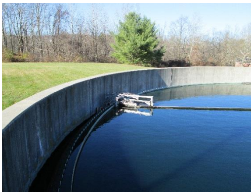
Final Clarifier – Weir Brush System
