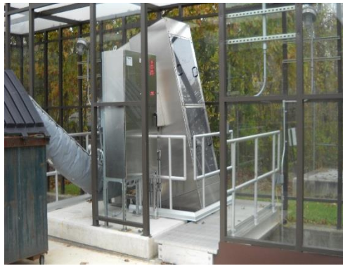
Raw Sewage Screen
