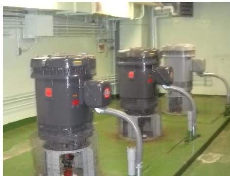
Raw Sewage Pump Motors
