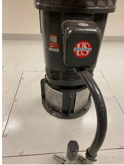
Raw Sewage Pump Motor with shield
