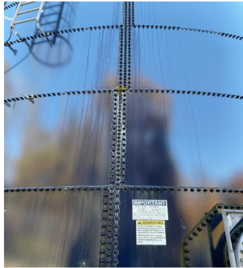
Independence Water Storage Tank Growth observed at Joint
