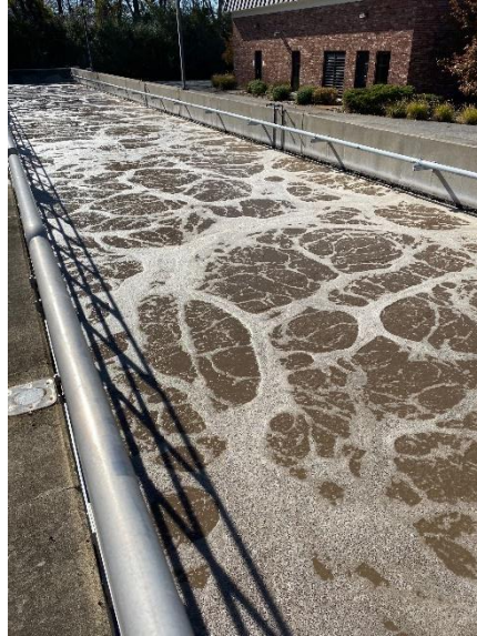
Nitrification Tanks with New Diffusers
