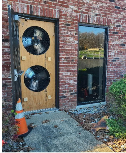
Blower Room – Positive Pressure System
