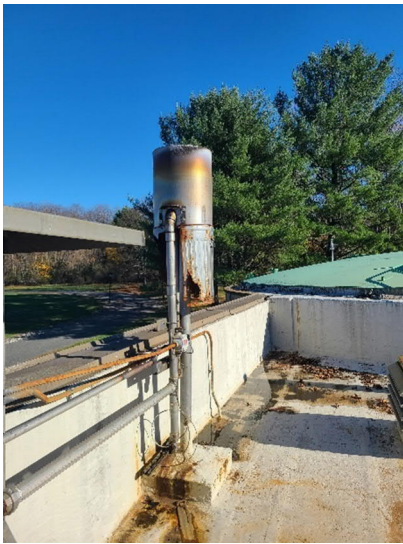
Flare on roof of Digester Building
