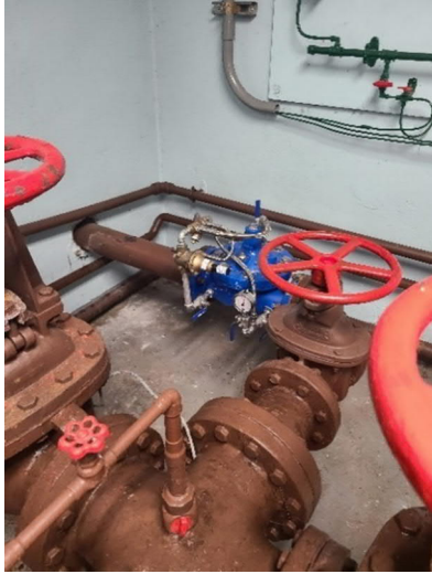
Well No. 4 – Altitude Valve
