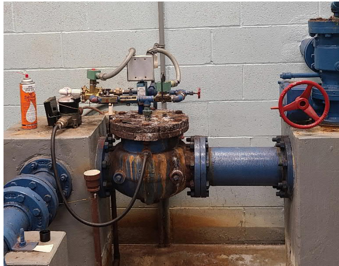
Independence Booster Station – Altitude Valve
