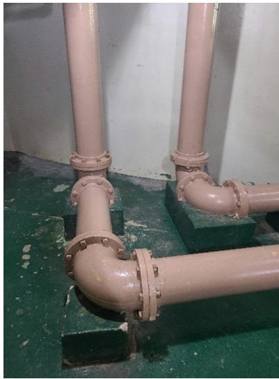
Digested Sludge Piping
