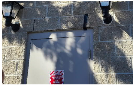
Yellowjacket entry to nest above door – duct tape
