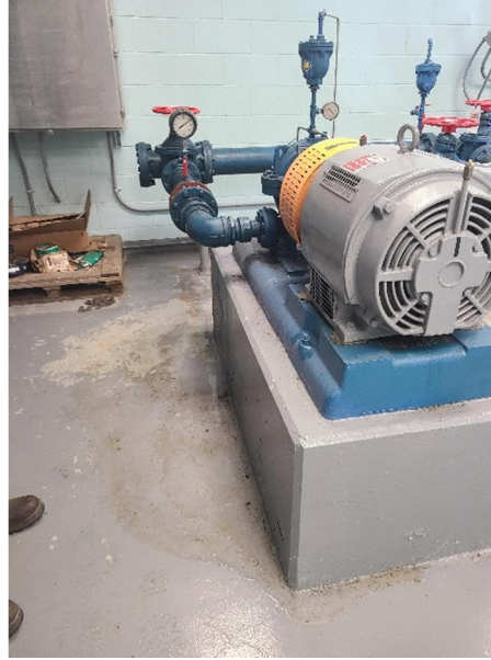
Mount Olive Booster Station Pumps
