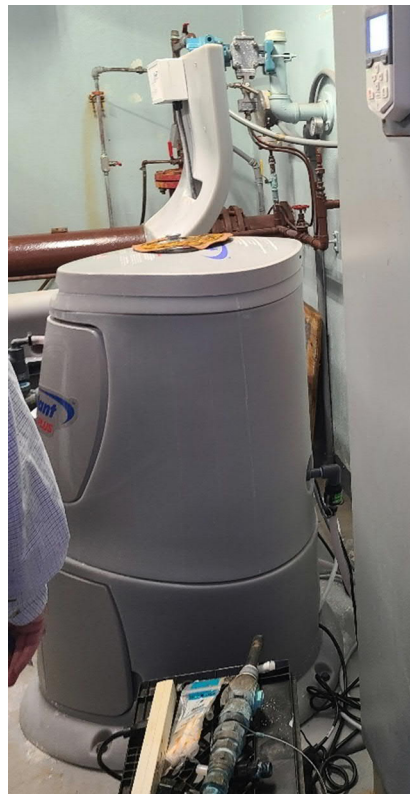
Chlorine Tab System
