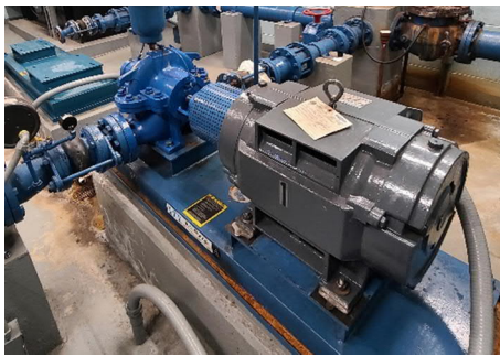
Independence Booster Station – Pump #1
