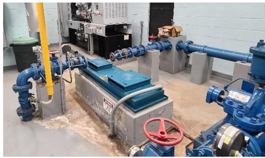
Independence Booster Station – Pump #2
