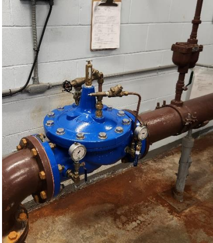
New Check Valve
