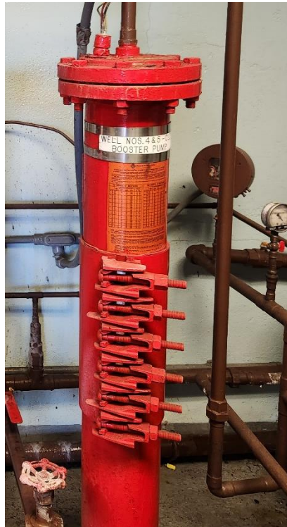
Well No. 4 – Booster Pump
