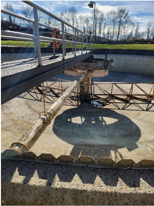
Intermediate Clarifier No. 2
