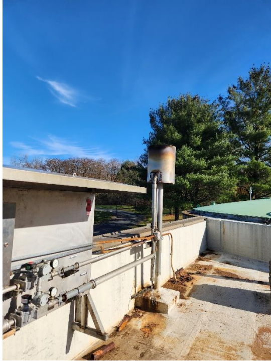
Flare on roof of Digester Building
