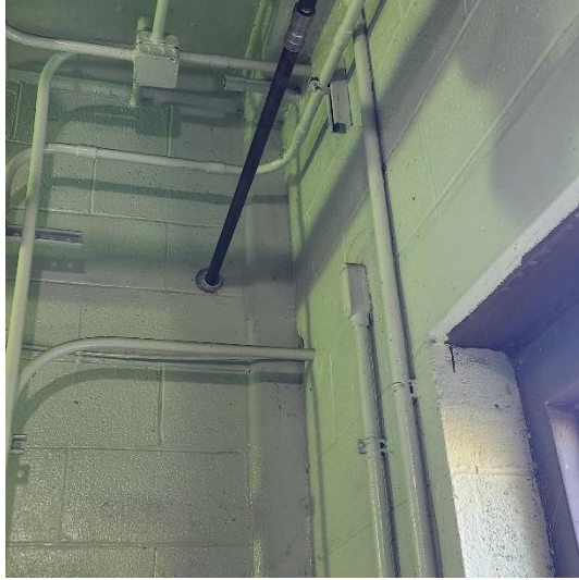
Piping for Flare
