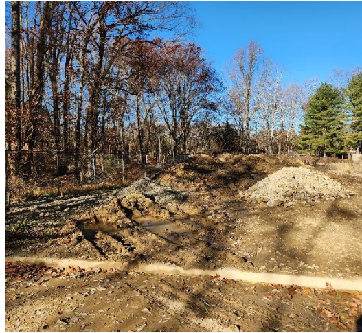
Stockpile and Damaged Fence
