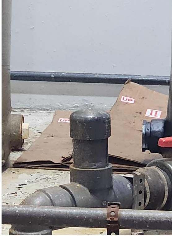
Fixed Alum Tank Leak
