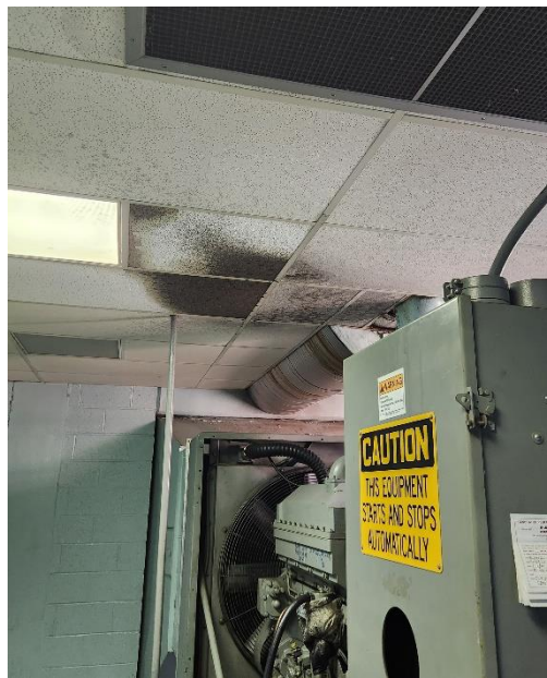
Damaged Ceiling Panels - Old Generator Room
