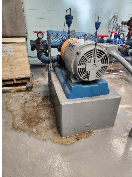
Mount Olive Booster Station Pump and Spare
